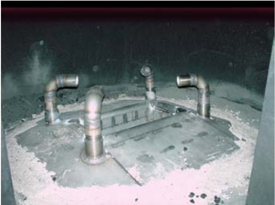
Fig.5: New stainless steel grate.
