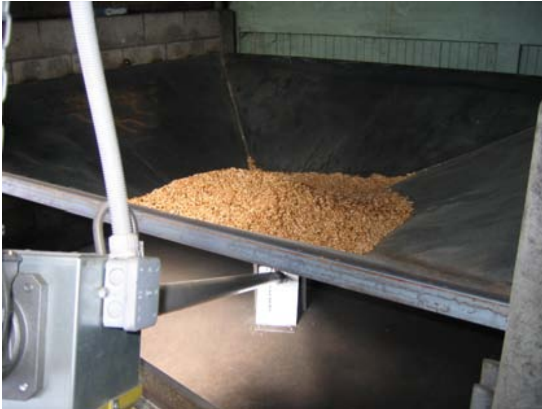
Fig. 7: Constant flow of wood pellets by coreless auger fed by steel bunker
