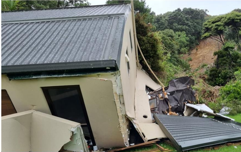
This photo of a house damaged during Cyclone Gabrielle clearly shows the exposure of EPS insulation to the environment. Photo credit: Tom Taylor, RNZ.
