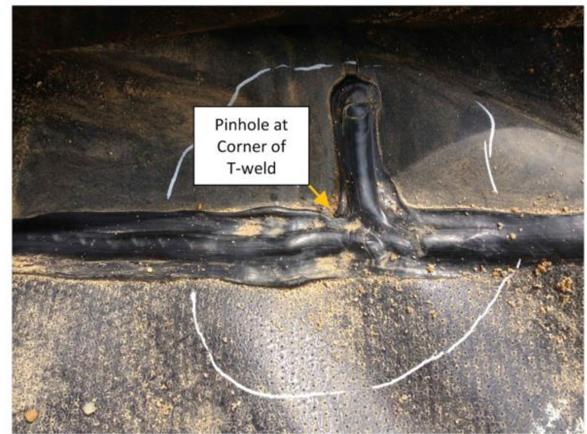
Fig. 8. One repair patch location with pinhole leak.
