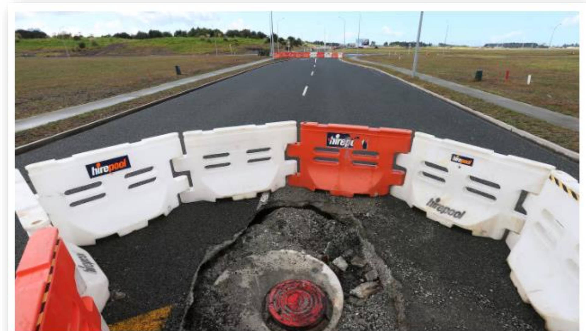
Subsidence in the Marsden City development could cost ratepayers millions to fix. Photo / NZME
